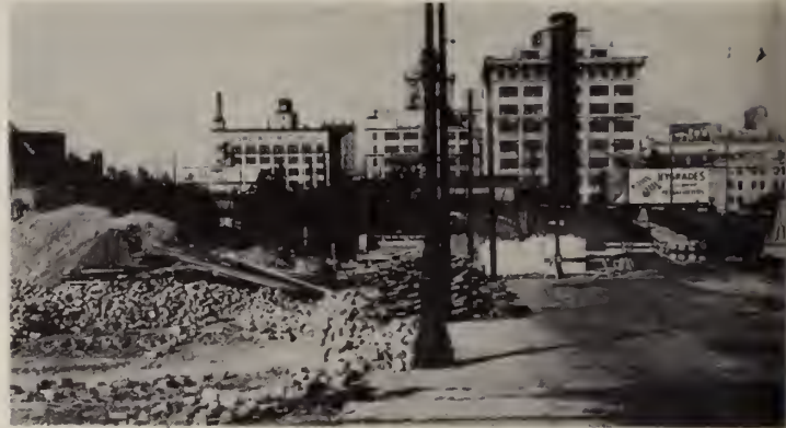
The Bridge approach prior to reconstruction, excavation for north roadway in progress.
